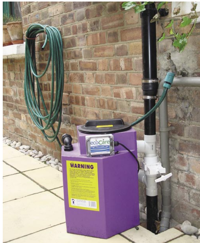
The Watermatic system diverts greywater directly to drain during the winter months; in the summer, when the greywater is required, it is filtered and pumped immediately to the garden so there is no chance of anaerobic decomposition.
